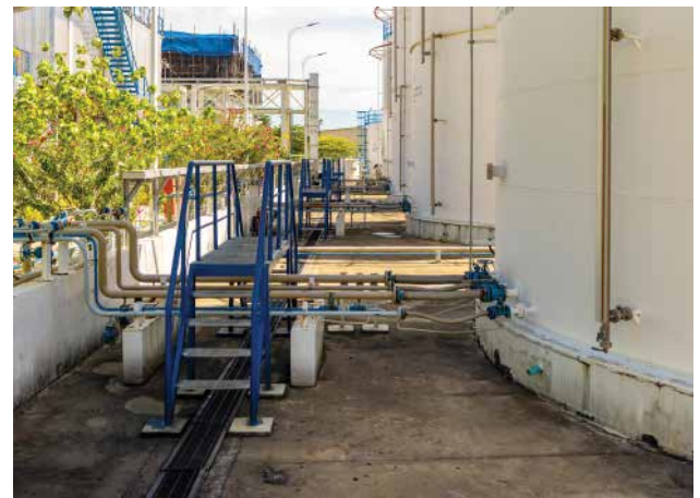
Figure 9 - Hulhumale Fuel line connections
