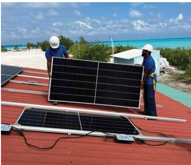
Figure 18 - K. Gaafaru Powerhouse, rooftop Solar Installation
