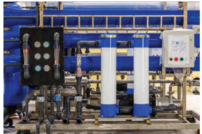
Figure 6 - Water Supply Facilities at K. Thulusdoo
