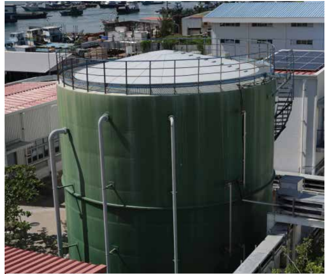
Figure 11 - Hulhumale' Water Storage tanks
