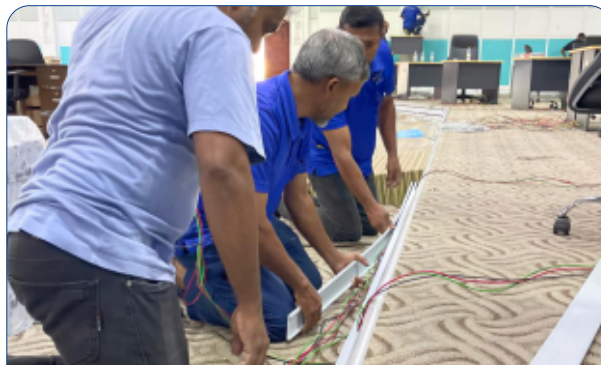
Temporary Workstations Setup Dharubaaruge - Dec 2024
